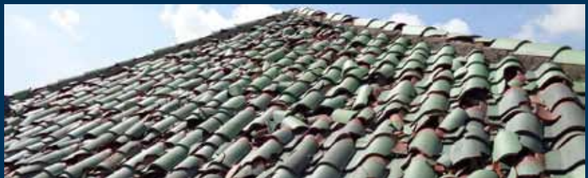
ROOF DAMAGE EVALUATIONS
